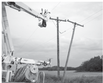
Linemen make repairs to a section of line on Hagan Road off of Highway 108 west of Carlinville.
